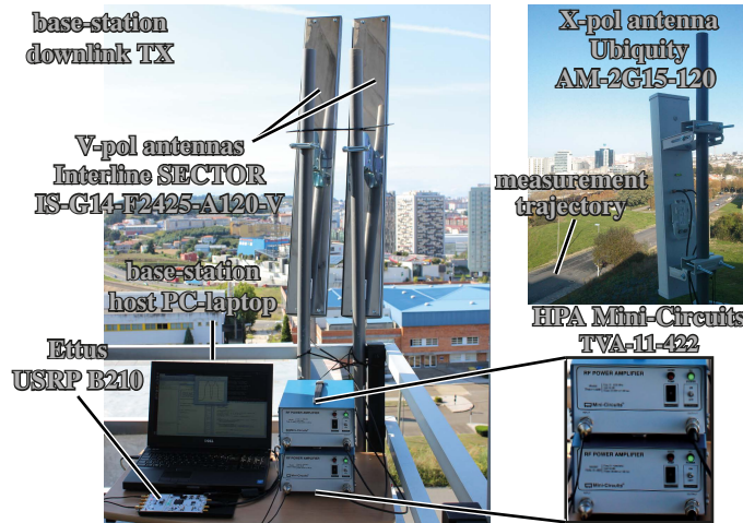
Figure 6.3: Base station downlink transmitter is placed outdoors, on the second floor of the CITIC building located in the Campus de Elviña at the University of A Coruña. Note that only one of the two vertically polarized antennas is used for 1 \times 1 transmissions, while both cross polarized antennas are used for the 2 \times 2 MIMO transmissions.
